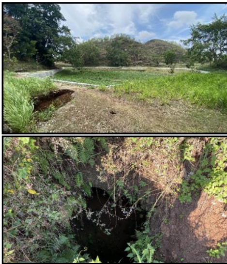
Figure 5. up, the sinkhole on the edge of Ngrinjing doline, and (down) the sinkhole that elongates at 2-3 meters
