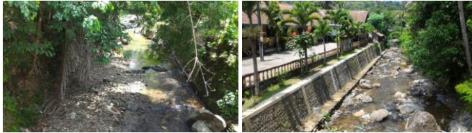
Fig. 9. Deposition on river bed at Loc.1.
