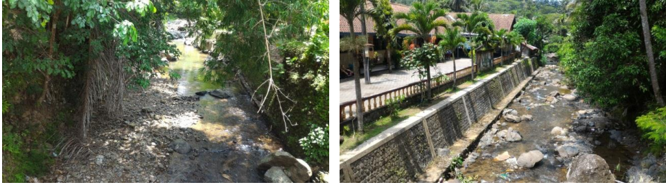
Fig. 9. Deposition on river bed at Loc.1.
