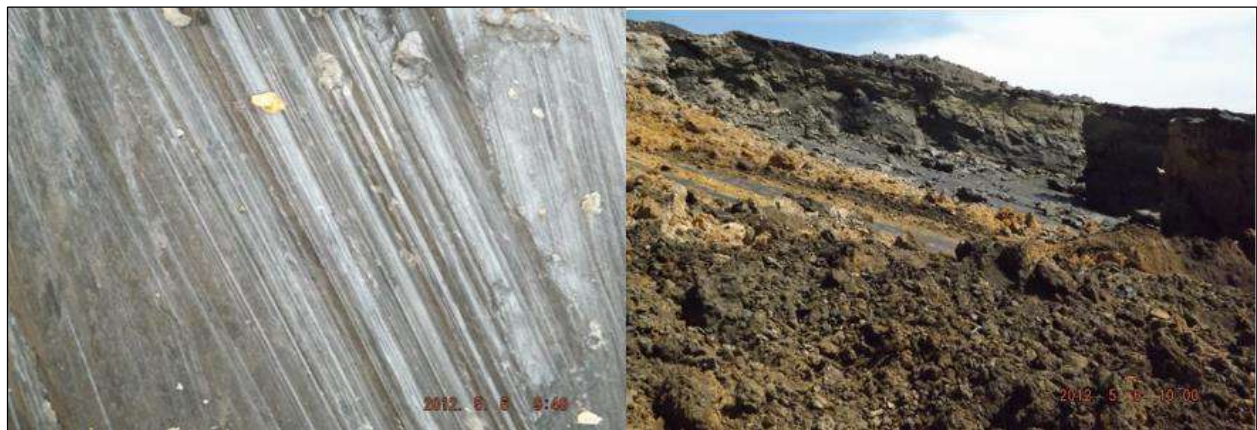
Figure 10. Slip surface on weak plane (left) and landslide at low-wall controlled by weak plane (right).
